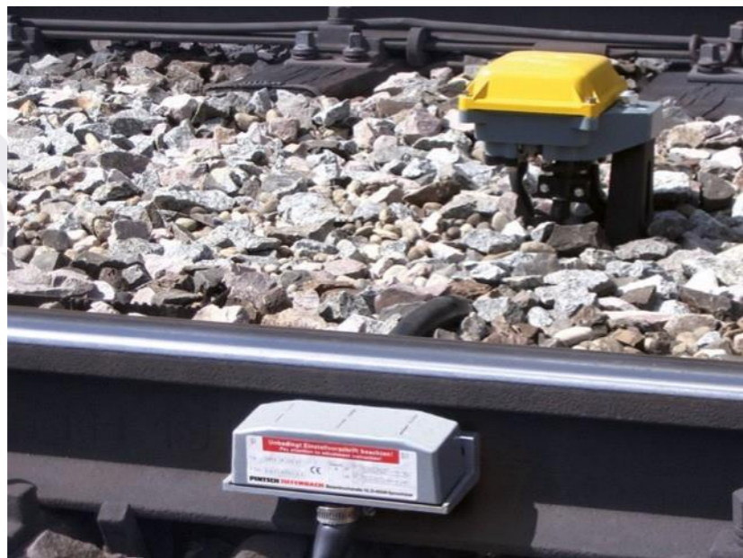
Figure 12 - Axle counter mounted on rail, and disbox (background)
