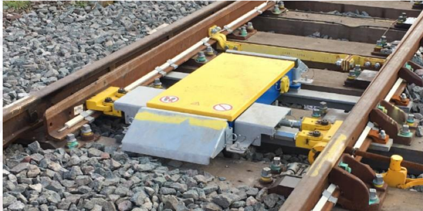
Figure 8 - Point machine installation
