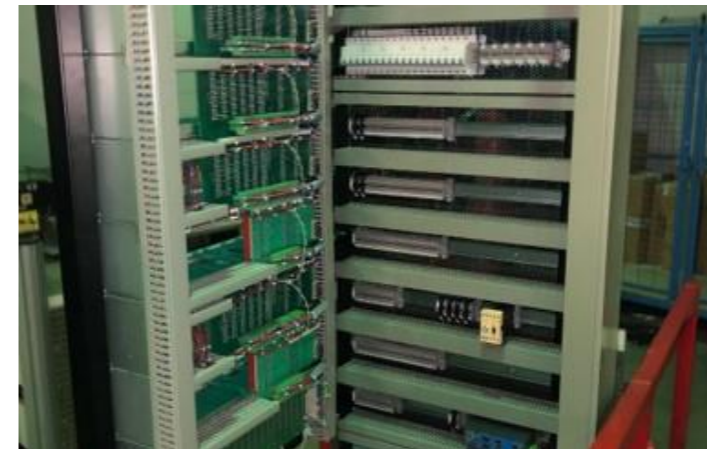
Figure 7 - Wall mounted internal location cabinet (undergoing factory testing)
