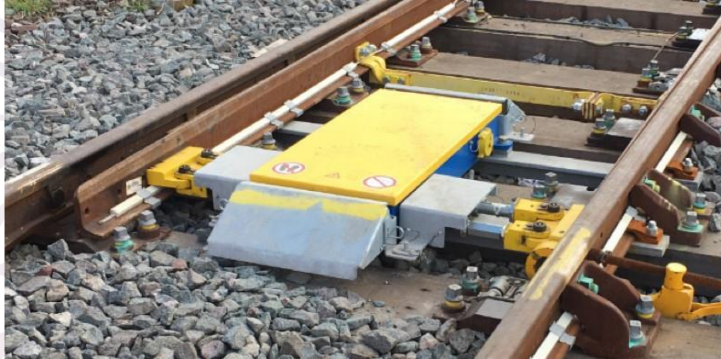
Figure 8 - Point machine installation
