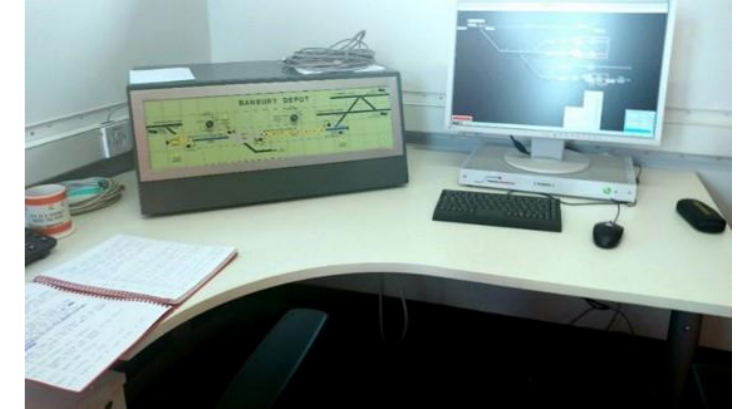
Figure 11 - VDU at Banbury Depot, UK (NR slot panel to left)
