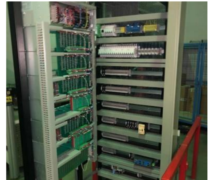
Figure 7 - Wall mounted internal location cabinet (undergoing factory testing)
