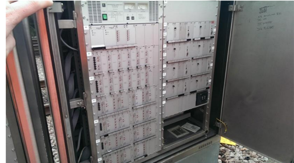
Figure 3 - Interlocking cards (Wembley Depot, UK)
