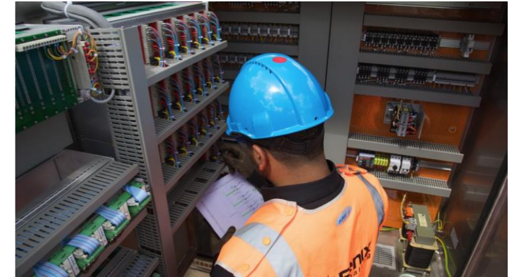
Figure 6 - External location cabinet (frame open)
