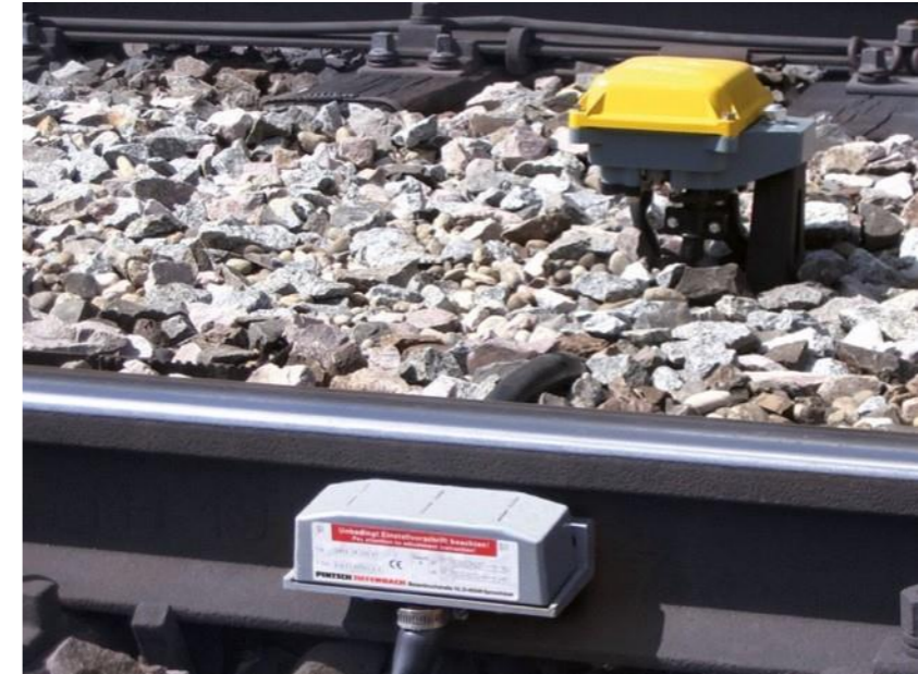
Figure 13 - Axle counter mounted on rail, and disbox (background)
