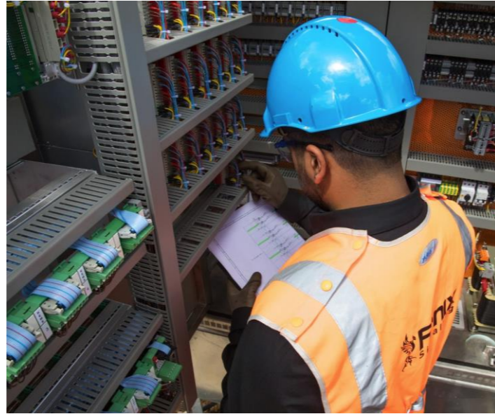
Figure 3 - Location cabinet (frame open)
