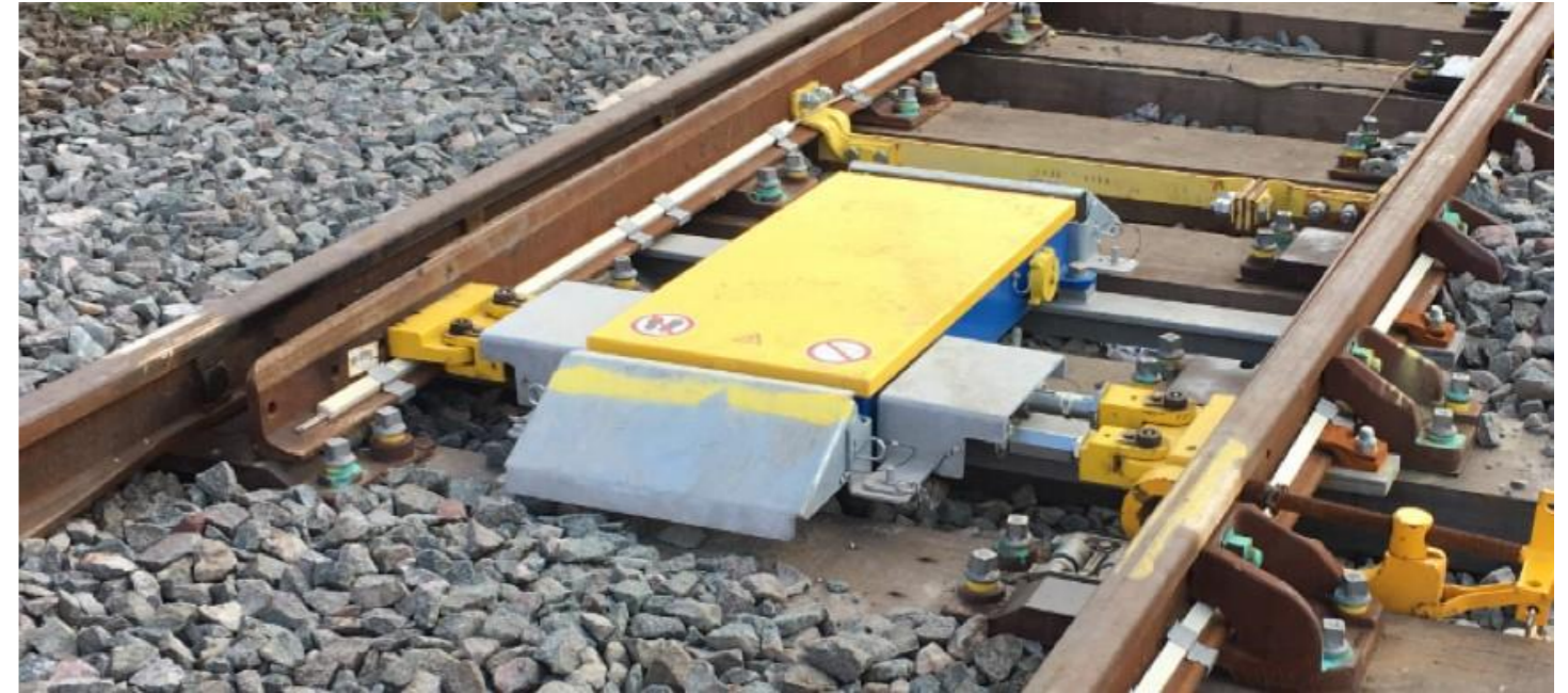
Figure 4 - Point machine installation
