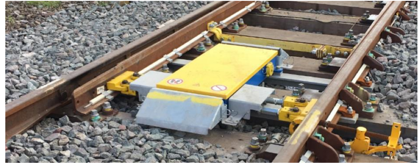
Figure 4 - Point machine installation
