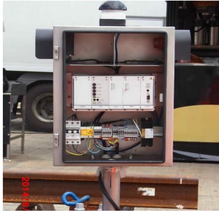
Figure 3 - Small cabinet with equipment for one point end
